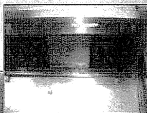
• Air duct and hood are still in clean condition 風槽及煙罩內能仍然保持清潔
